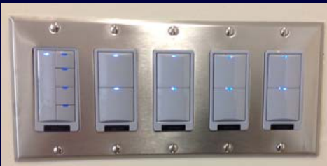
Classroom Wall Switch
